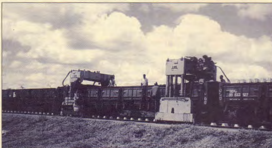
The Beitbridge-Bulawayo Railway is one of the projects in which the private sector have successfully participated.
