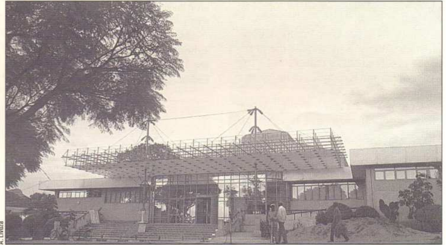
GETTING READY: This photo taken in June shows the finishing touches to the new Convention Centre in Blantyre, the venue for the SADC Summit
