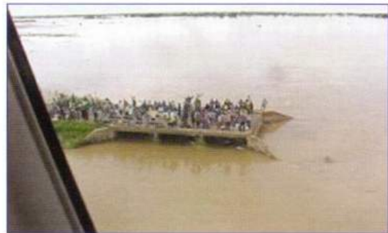
People stranded on a broken bridge
