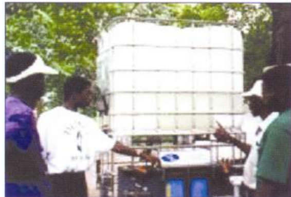
Water purification plant donated by UMCOR
